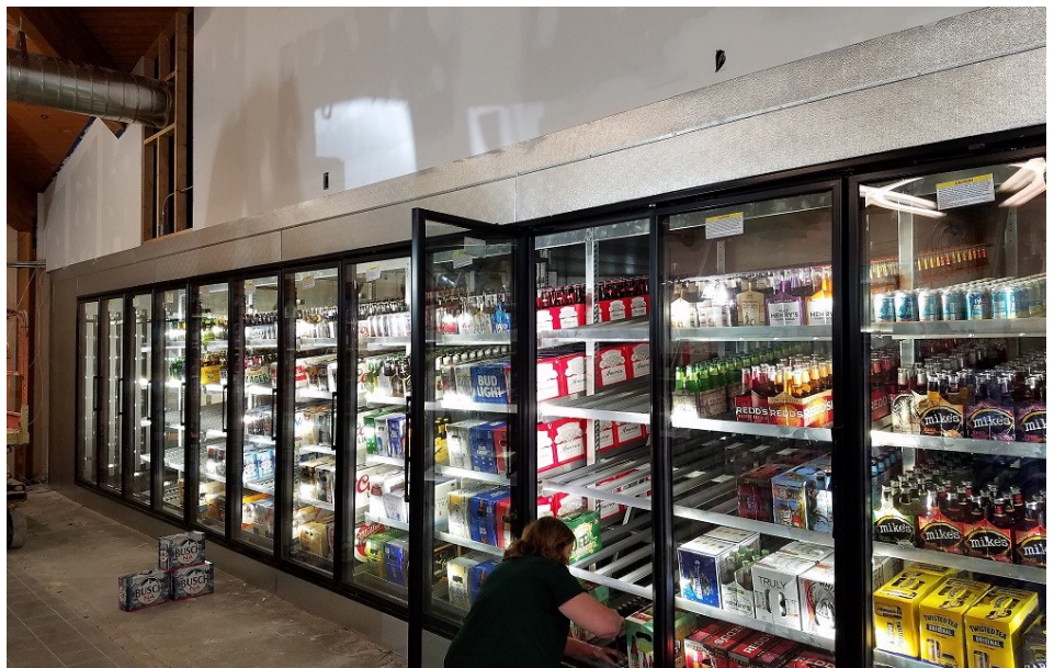
New Cooler at Liquor Store
